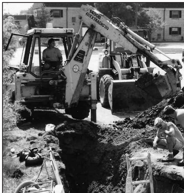
Public Works crews replace a section of underground water main. The City's system contains more than 90 miles of pipes, which deliver nearly 15 million gallons of water to customers each week.
