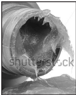
FOG buildup will eventually cause sewer backups and overflows.
