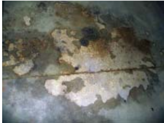
Parking Bay Floor Delaminating
